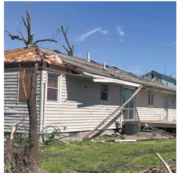
Joceline and Curtis Vry's home was severely damaged in the May 21 tornado that hit Greenfield.
