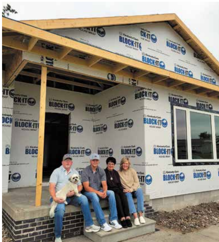
Jennifer and Jeremy McDermott show their new home under construction. Pictured left to right: Jeremy holding Boomer, Kaden, Judy Jensen, and Jennifer.
