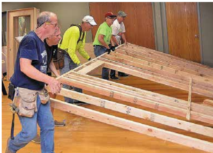
Members of Sacred Heart Parish in West Des Moines build a wall in the parish hall as a means of using their gifts to help others.
