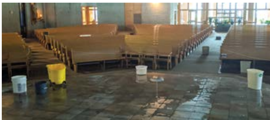
The interior of St. Pius X Church in Cedar Rapids, Iowa, is seen after the Aug. 10 derecho windstorm. A rubber covering on the roof was blown off causing water damage. (CNS photo/courtesy Michael Becker via The Witness)
