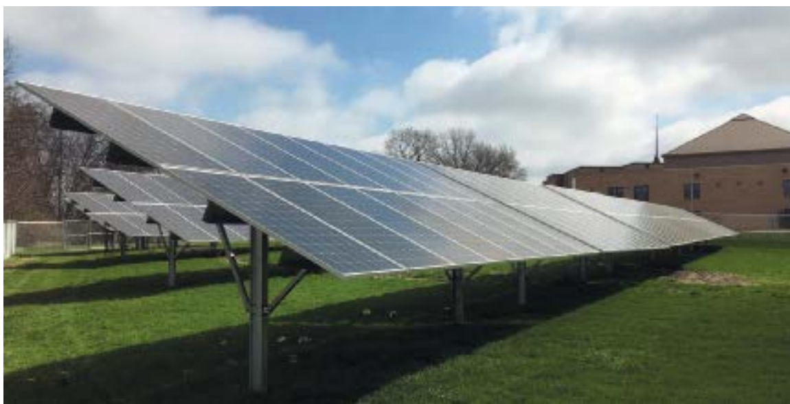
All Saints Parish in Des Moines recently installed solar panels to reduce the parish's carbon footprint and save money.
